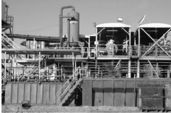
Shale shaker isolating drill cuttings from the drilling fluids.
